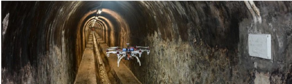
Fig. 3. Quadrator flight in Passeig Sant Joan in Barcelona, a real sewer environment.
