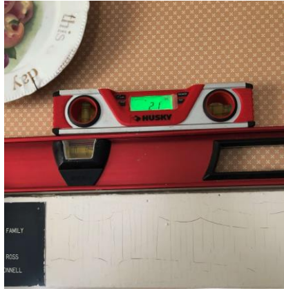
Figure 1. Plumbness of header above doorway
