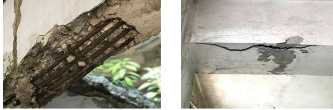
Fig. 1. Corrosion deterioration of RC beams
