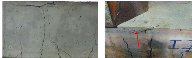
Fig. 8. Failure mode of D-1 and D-2 beams
