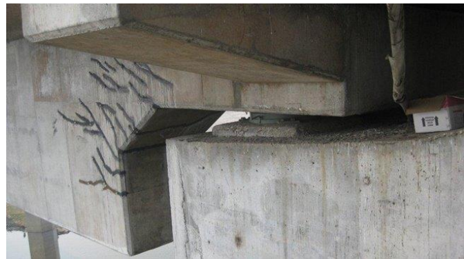
c) Cracks on Half-Joint
